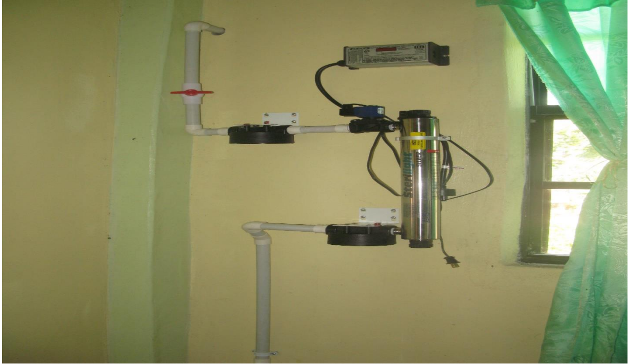
New water filtration system installed by Jonathan Moyer
